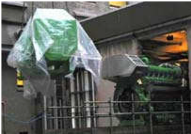
A CHP facility at the University
