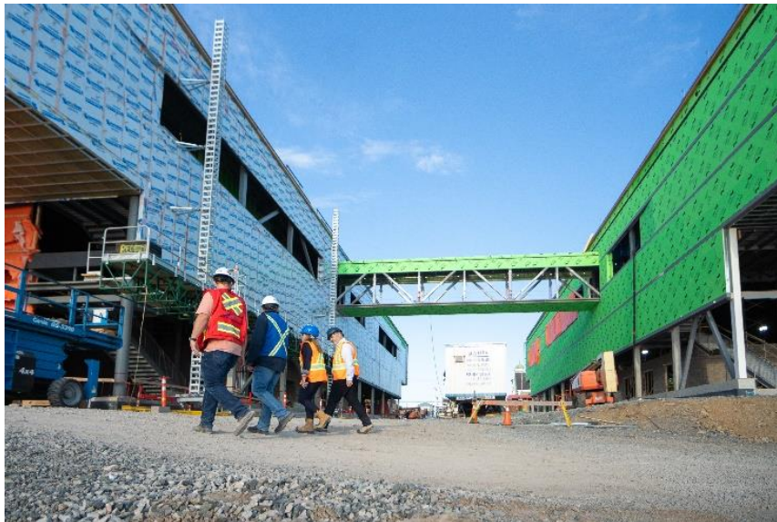
Construction at the new Sydney Waterfront Campus, our most sustainable campus to date
